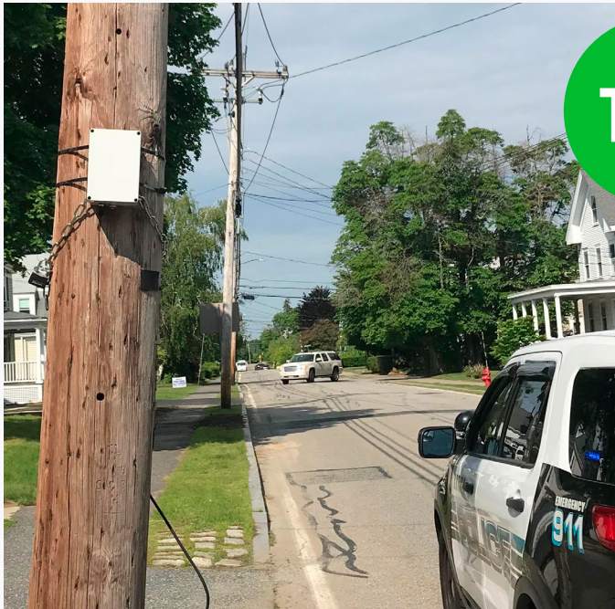
A StatTrak counter classifier mounted on a pole
