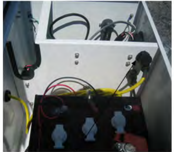
instALERT Power Plug in Battery Enclosure
